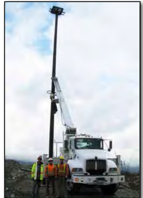
L to R: Mike Unger (Ridgedale Rod & Gun Club), Clayton Olivier (Owner of Valley Power Line Contracting), and Steve Abrahms (employee of Valley Power Line Contracting) after erecting a new 75' pole that will host the osprey nest.
